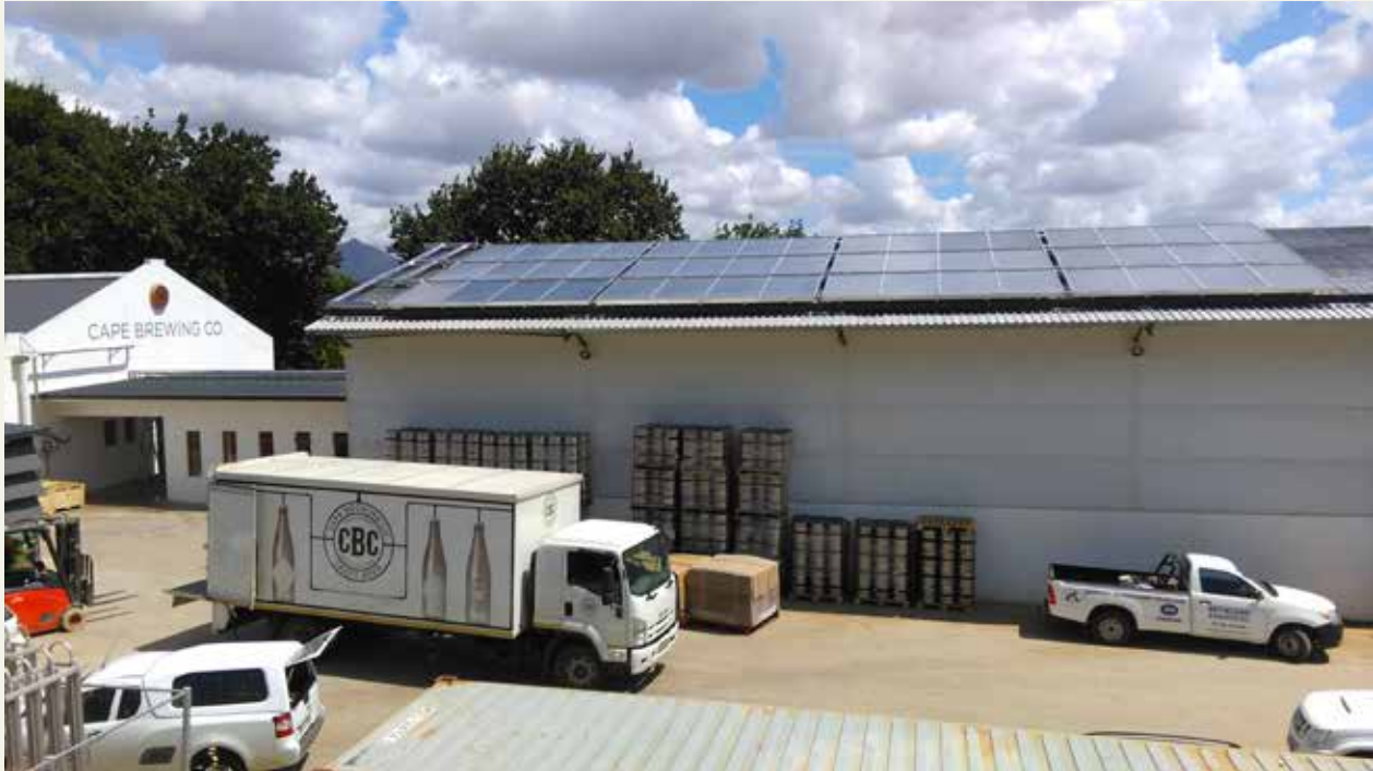
Figure 14: CBC brewery's 120 m 2 flat plate collector array
